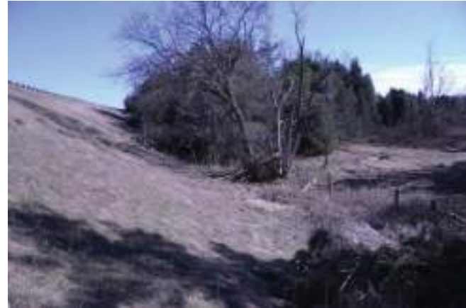
West slope of Highway 400 embankment. Culvert arch located behind woodlands in foreground
