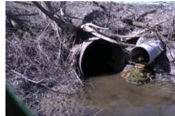
1.7 m diameter culvert conveying Innisfil Creek (left). Smaller CSP conveys flow from north ditch (across) – note deposits at outlet
